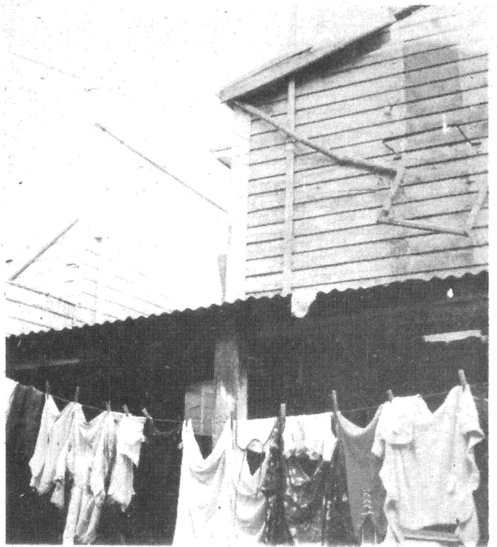
Illegal roofs — no spouting, bargeboards missing.
